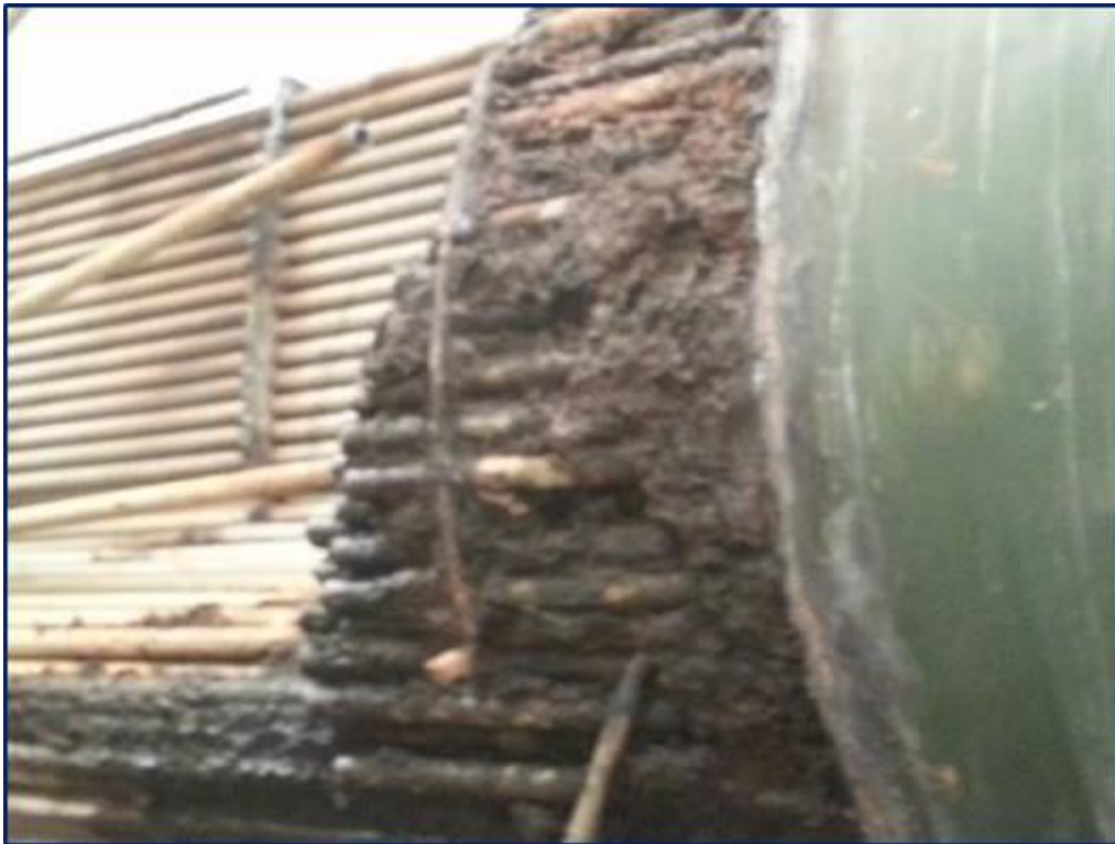
Figure 3: Old Heat Exchanger Corrosion
