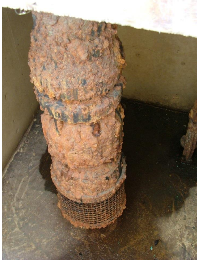
Figure 2: Old Cooling Tower Pipe
