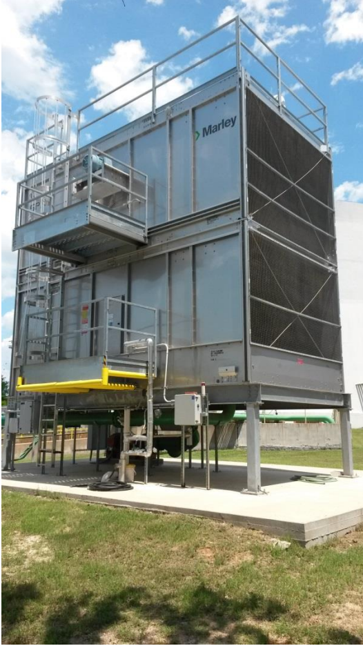
Figure 4: New Cooling Tower
