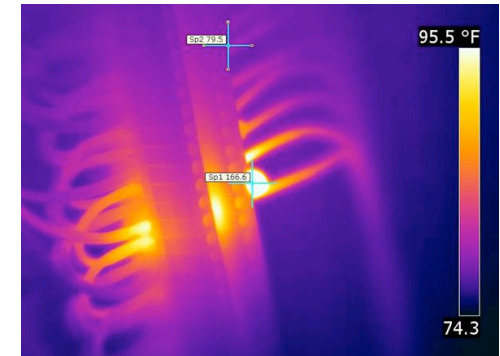
Cold Source Cold Box Wiring
